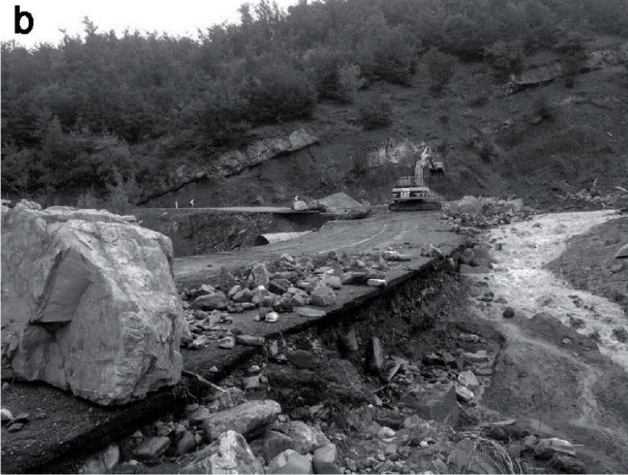
Rio di Confine, boulders with size of 5 m 3 deposited along the provincial road
